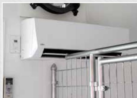
Interior View of Mini Split Heater/AC Unit
